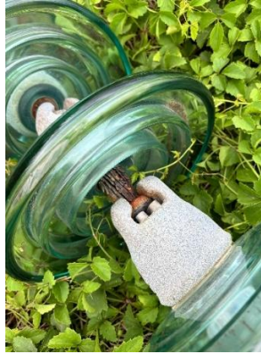
Gambar 1. Steel pin isolator korosi
